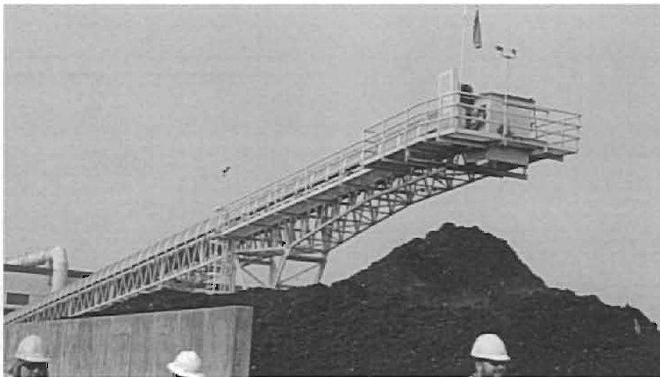
Mixed product coming from the mixing building – prior to being transported to the active phase ASP area.
