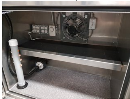
Example Pump mounting cabinet with exhaust fan
