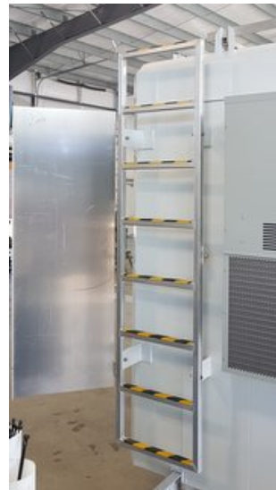
Ladder access with cover
